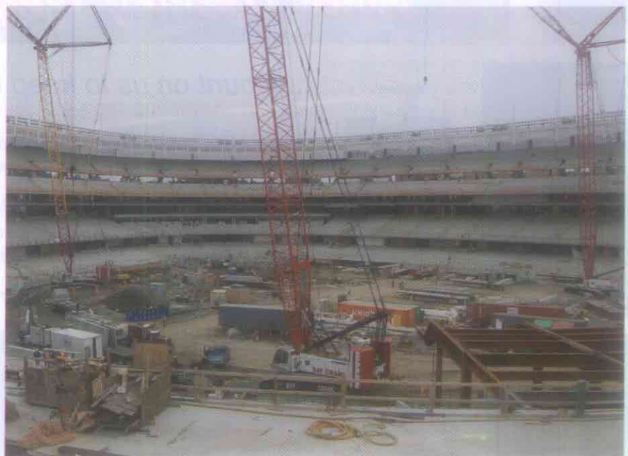
Staging has been difficult on the Yankee Stadium site, which is surrounded by a subway line, a residential street, the existing stadium, and a park. Photo by Andrew Wright.
