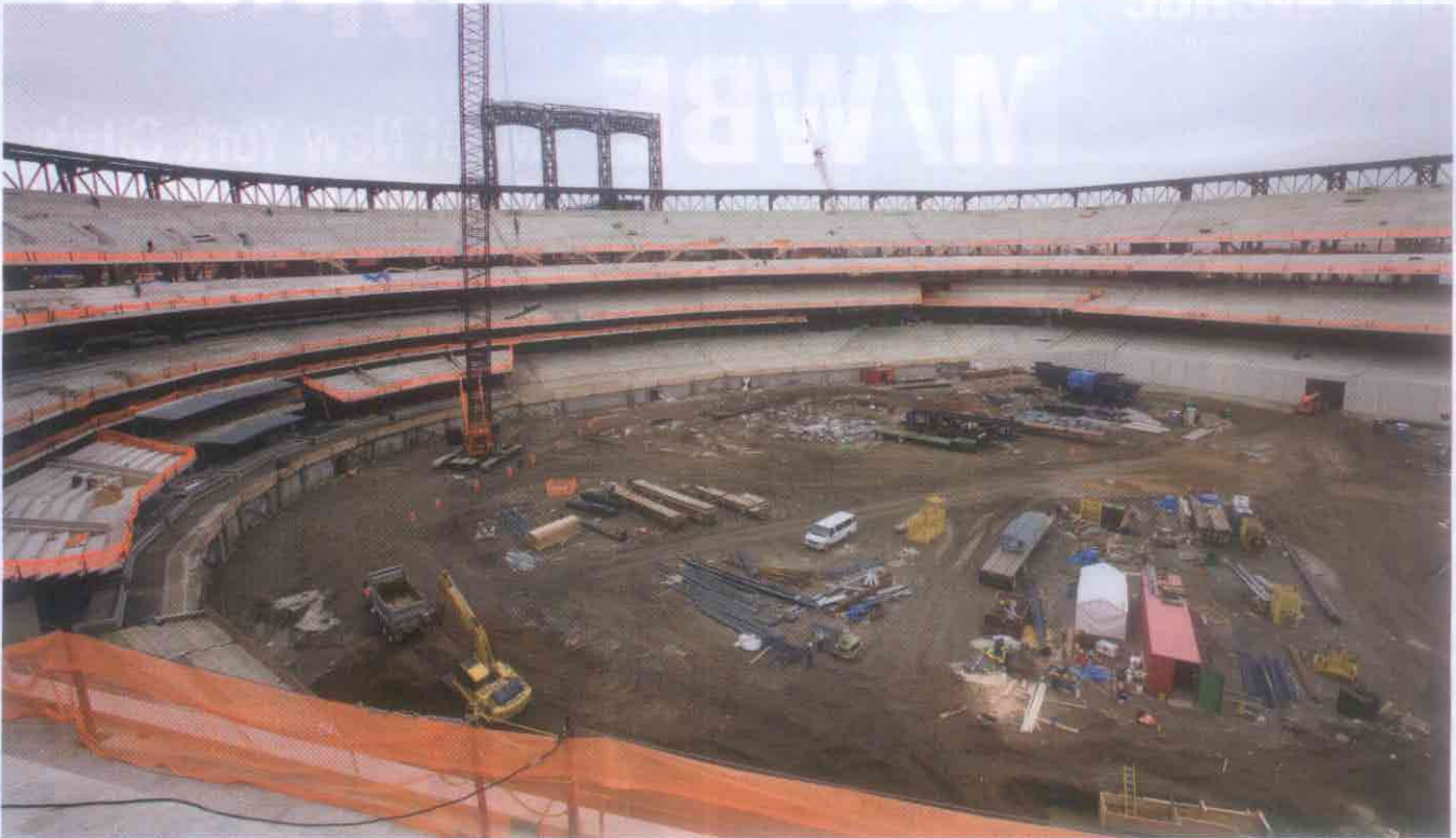
With most of the high work completed in early spring, the focus now is shifting to the lower seating bowl, which will start at the ground level. Note: Home plate is surrounded by the orange fencing to the right of the crane. Photo by Michael Falco.
