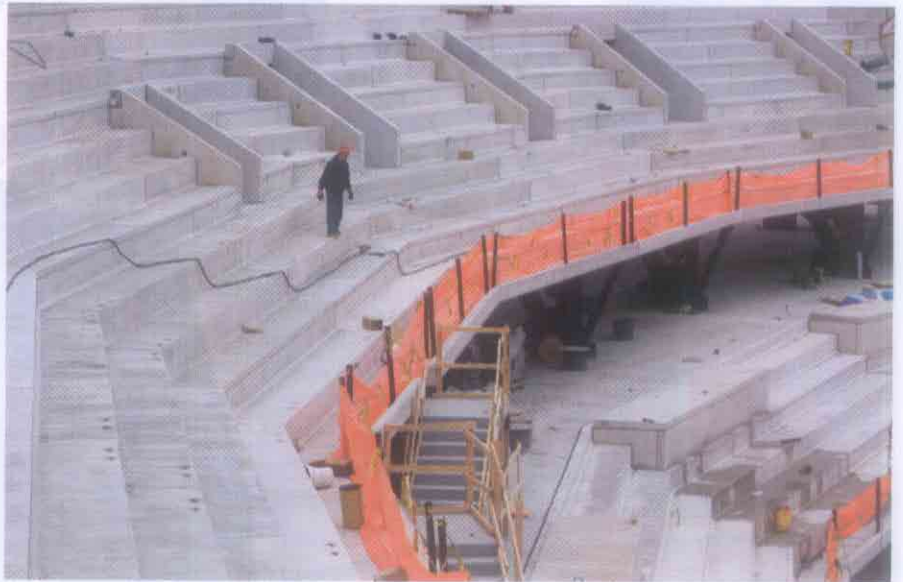
In March, crews at the Citi Field site in Flushing began installing the first of the stadium's 45,000 seats in the upper deck. Photo by Michael Falco.
