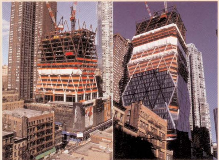
Hearst Tower at 57th Street and Eighth Avenue
